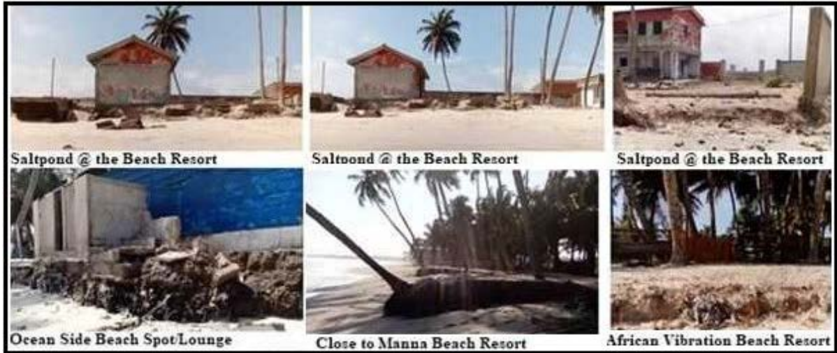
Figure 1: Photographic Evidence of the Destructive Impact of Sea Erosion along the Coast of Saltpond.
